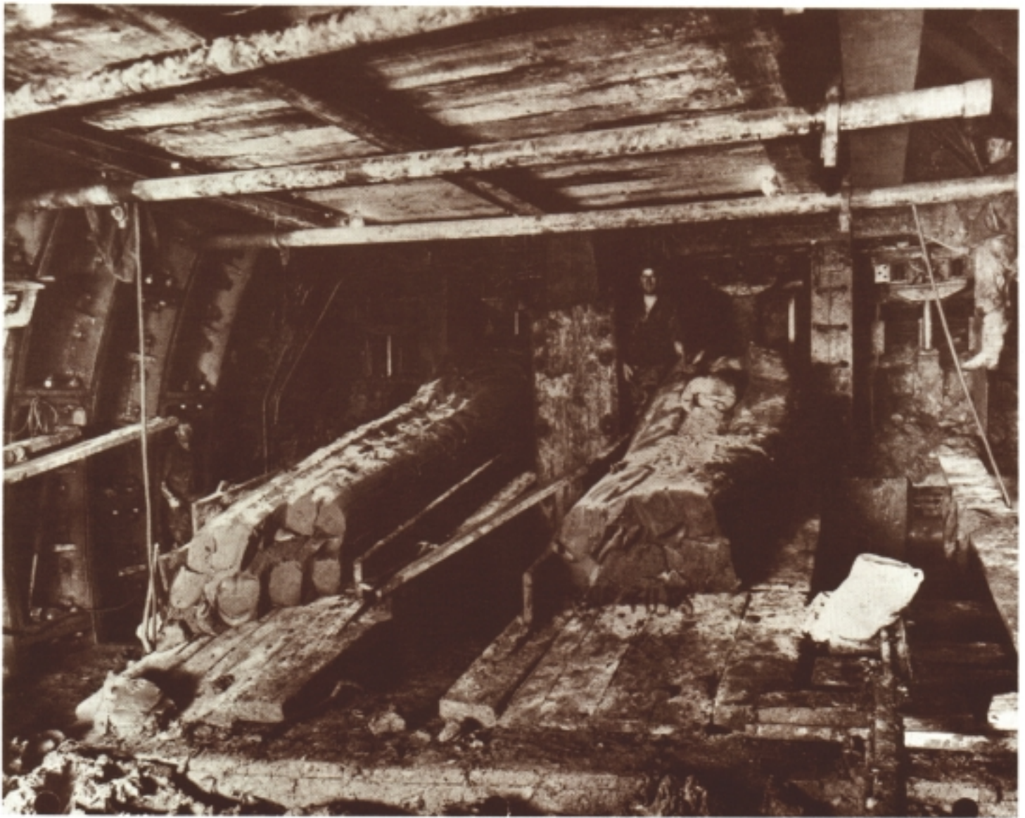
VIEW TAKEN DURING A SHOVE IN THE SOUTH TUNNEL EAST, JERSEY CITY, SHOWING SILT FLOWING INTO THE TUNNEL THROUGH SECOND LEVEL POCKETS.
