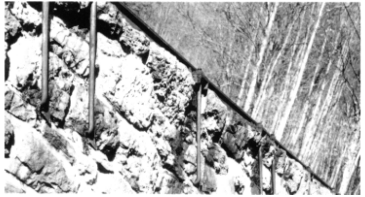
The iron ties (of the bow bridge) go through the wall of the bridge.
