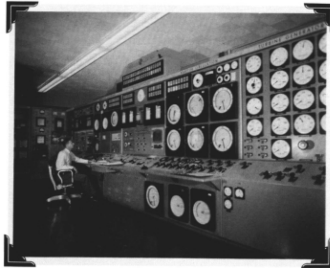
Reactor control panel.
