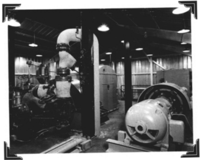
Interior of turbine-generator building.
