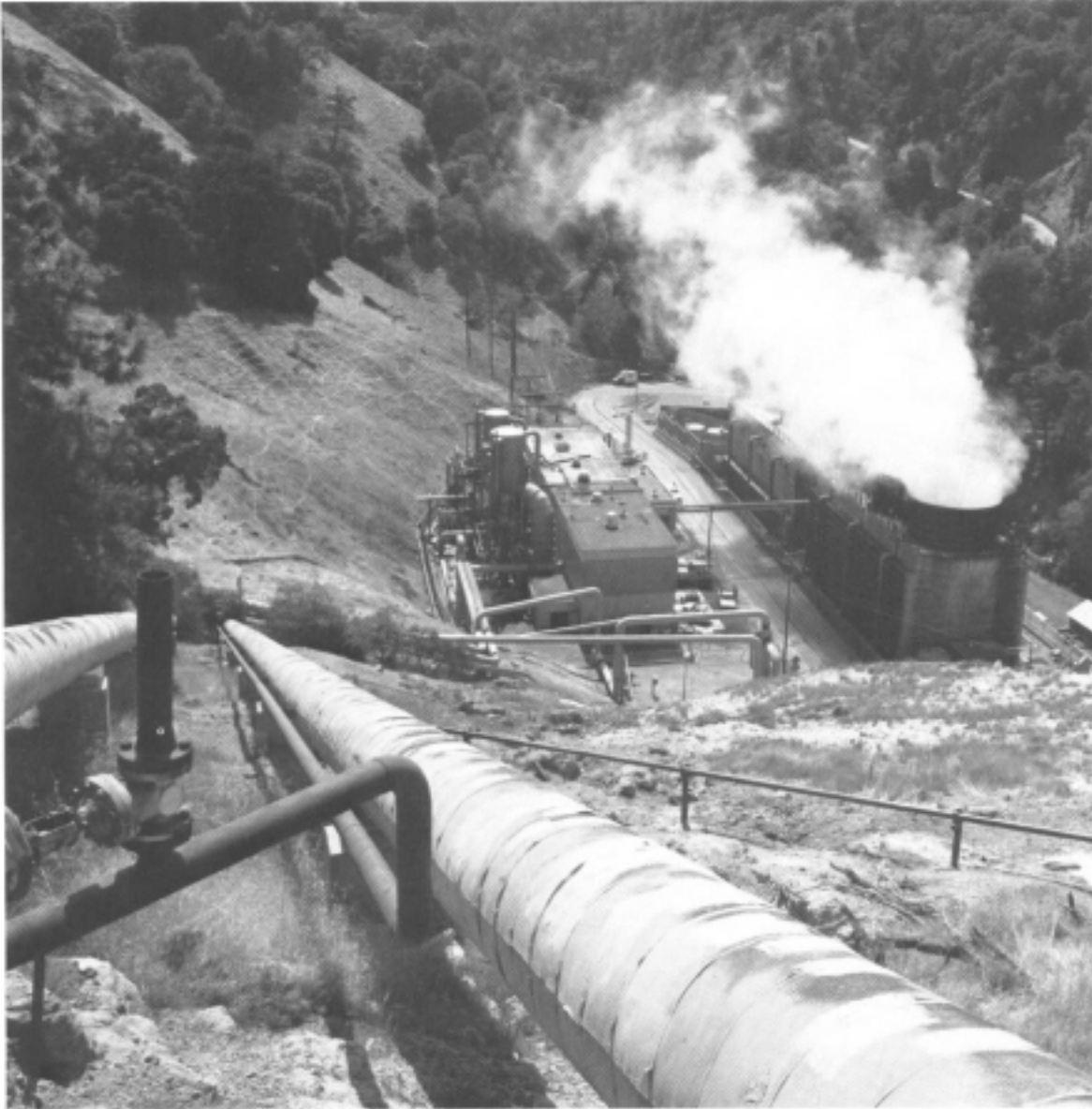
Unit I, the grandfather of geothermal energy in the United States, continues to produce power at The Geysers. Today it sits in its hillside home next to Unit II.
